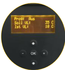
Digital control panel
